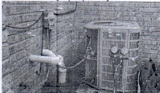
Valve and gauge (25/05/2016)
